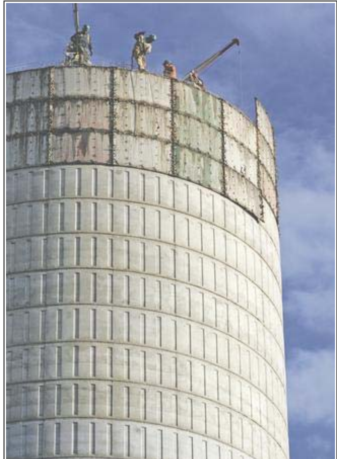
Crew members work on an elevated water storage tank being constructed off Rocky River Road Thursday.
